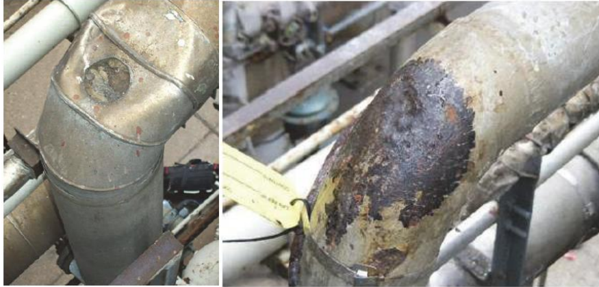
Pic p4—Jacketed piping with missing insulation plug (top photo) allowing water ingress. Ref-API 583
